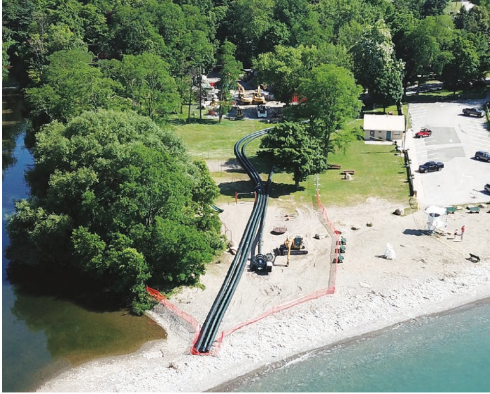
HDPE pipe on the beach.
